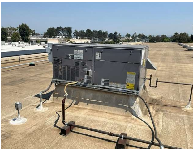
15 - ROOF TOP UNIT
