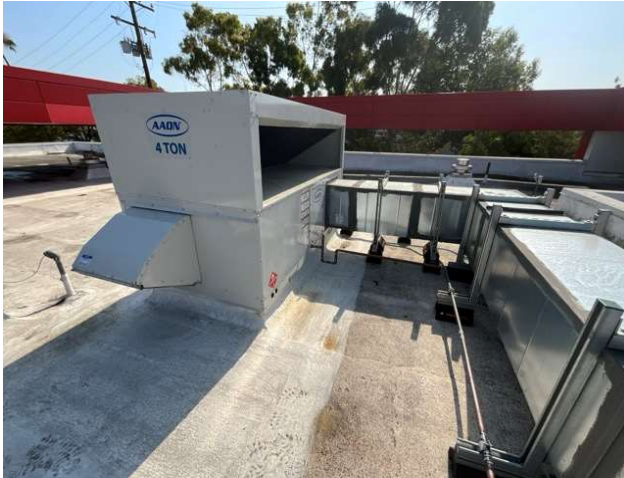
13 - ROOF TOP UNIT
